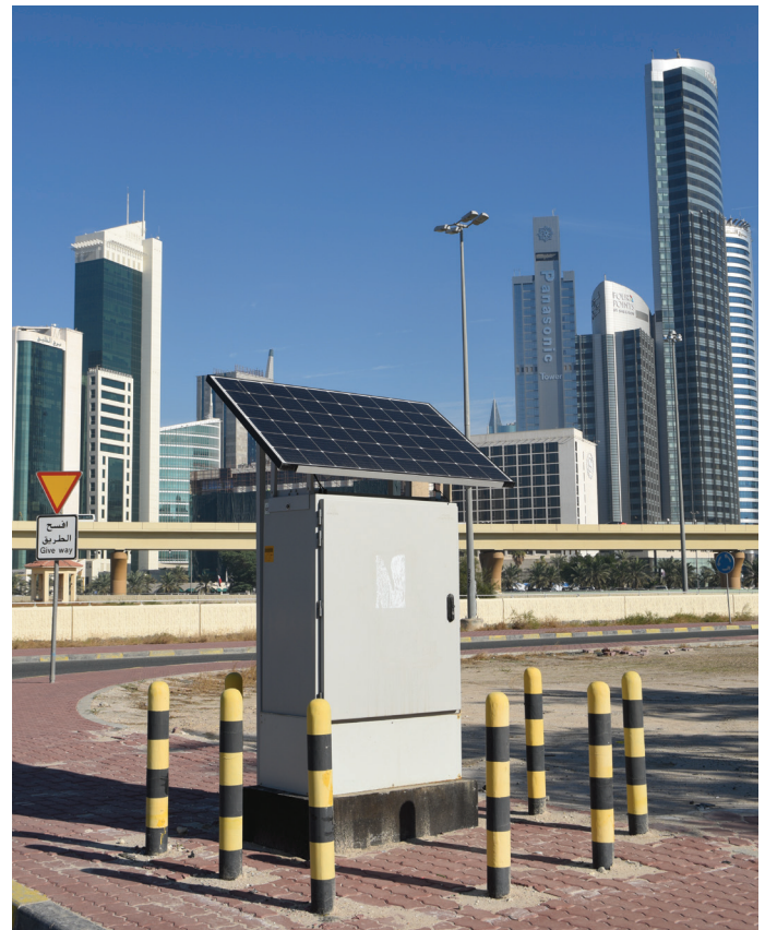
Figure 4: A complete solar-powered measurement station.
