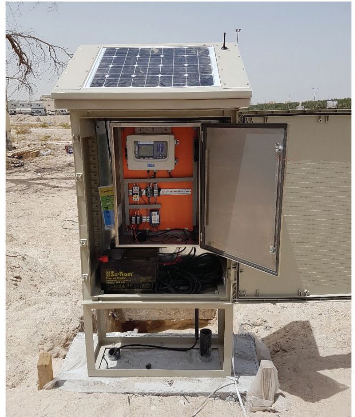
Figure 1: Teledyne ISCO LaserFlow demo installation in Kuwait City.
